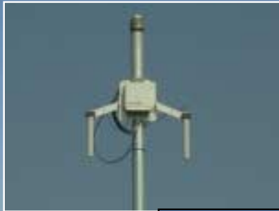
On pole behind freight house
